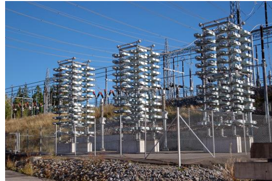
Figure 1. An ABB shunt capacitor bank.
