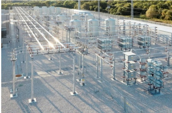
Figure 1. ABB static var compensator outside Dallas, US. The three long parallel conductors in the left part of the photo shows an example that have motivated the conductor setup considered in this project. Picture by ABB.
